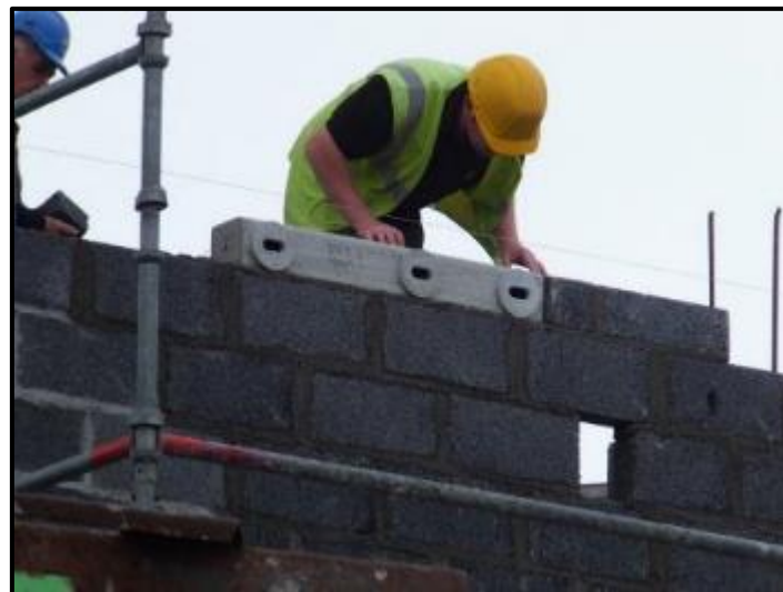
Figure 25: Installing Swift boxes as part of the fabric of the wall. Photo: Lynda Huxley
